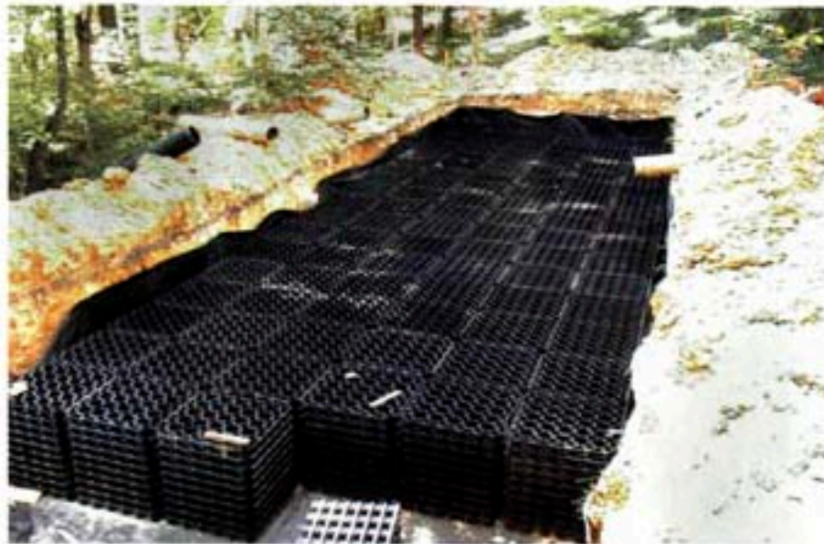
A large infiltration pit was built to collect runoff, allowing it to seep into the soil rather than directing it off the site as the existing drain pipes had done.
