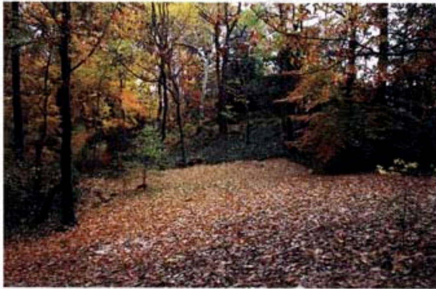
The completed infiltration pit is not visible to Olmsted Woods visitors, in keeping with the naturalistic aesthetic of the site.
